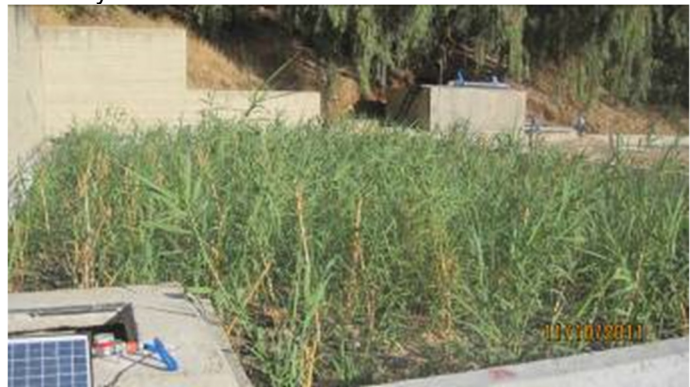
Sludge bed 2 months under operation
