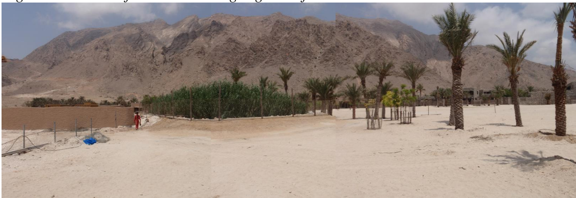
Sludge mineralization reed bed for Six Senses Resort in Zighy Bay, Oman (300 cbm sewage per day)
